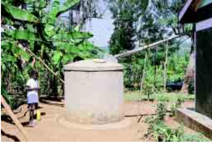
Ferro cement tank of around 5,000 litres, constructed by Katuntu Tweekembe Women's Group at Nalongo Kikomoko's homestead.
