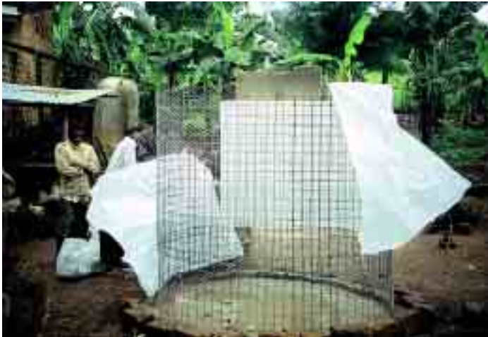
Tank construction under way. The base has been built and the tap fitted. The wire mesh is being put in place.
